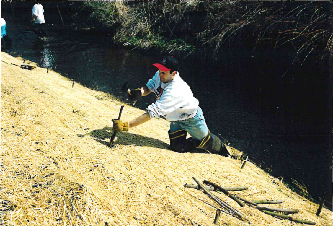
Installation of Live Stake (Note rubber mallet being used to tamp stake into place.)
